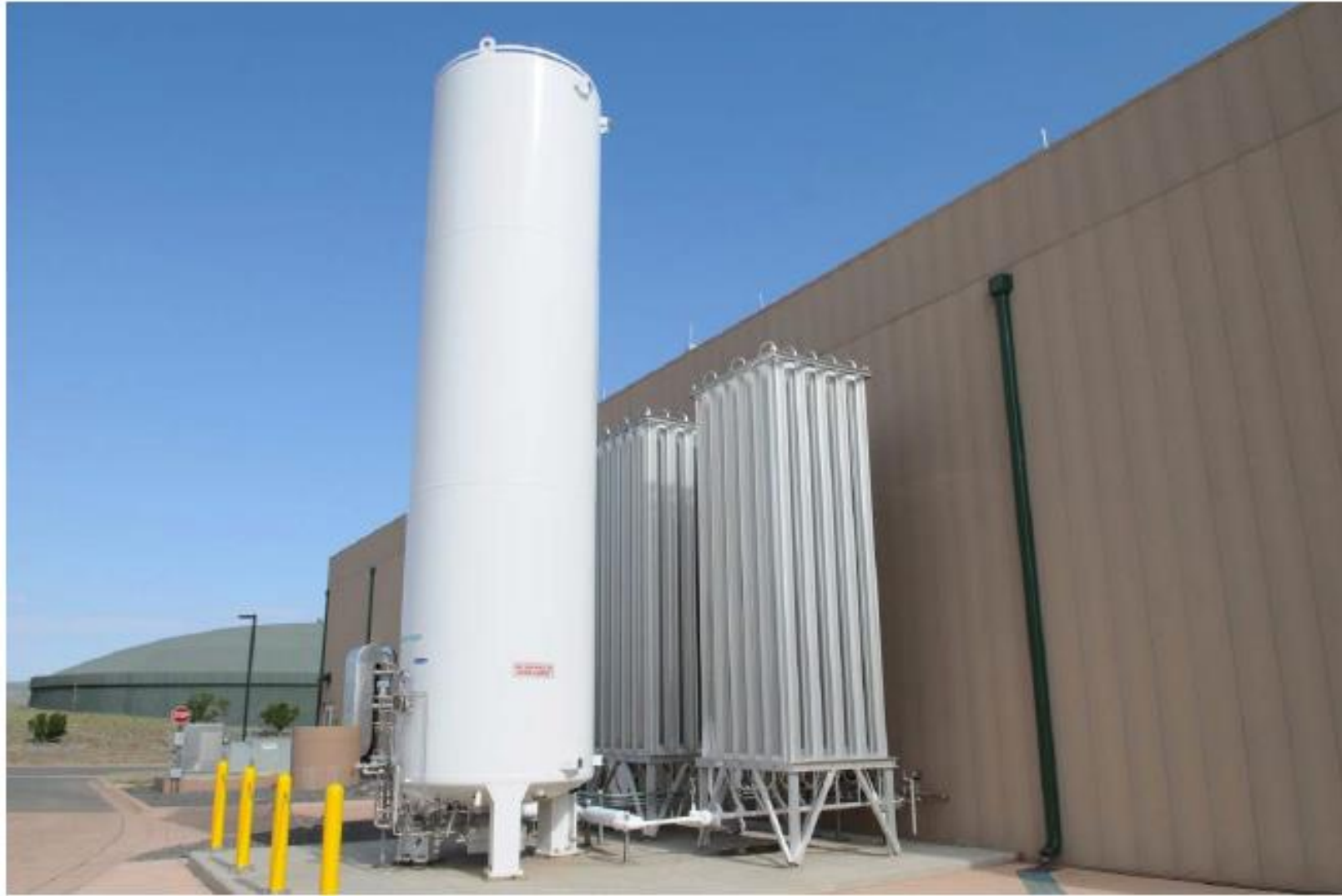
Figure 18. An Existing Liquid Oxygen Storage Tank and Vaporizers. Liquid oxygen deliveries would include delivery of 20 tons of oxygen every two and a half weeks.
