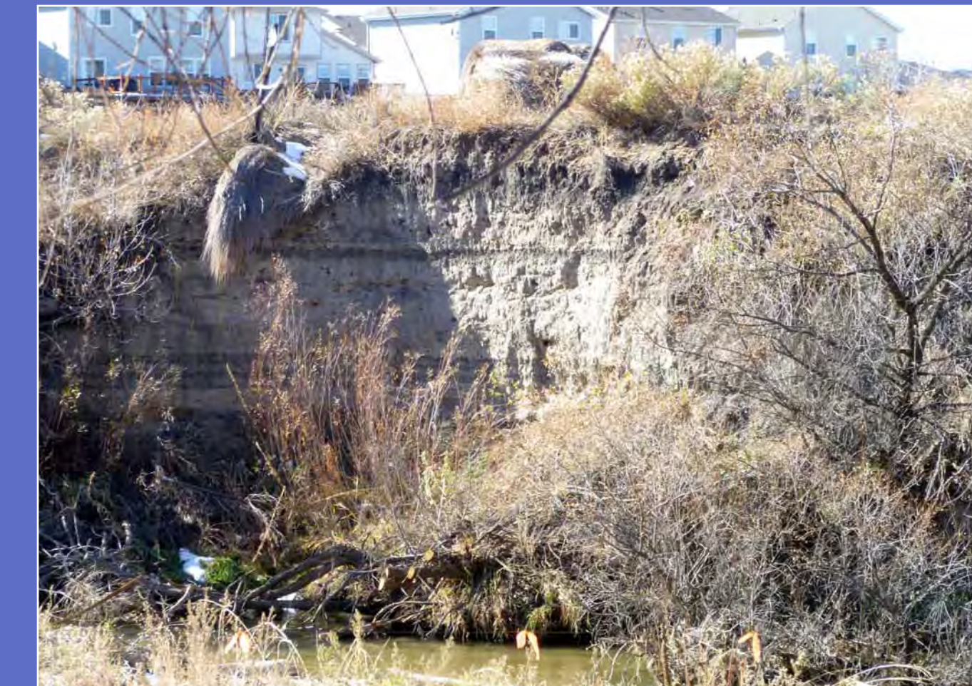
A picture of the dramatic bank erosion found along Cherry Creek at Parker Jordan Centennial Open Space prior to reclamation.
